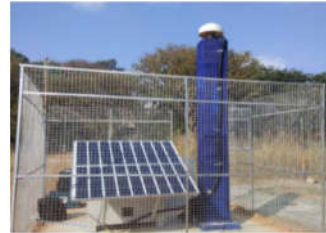
CORS Station Setup
